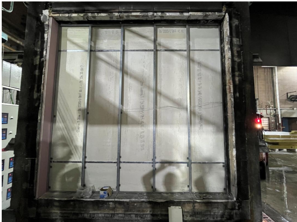
Photo 2 - Specimen during construction - Unexposed side boarding view from exposed side. Note the angles on the horizontal joints.
