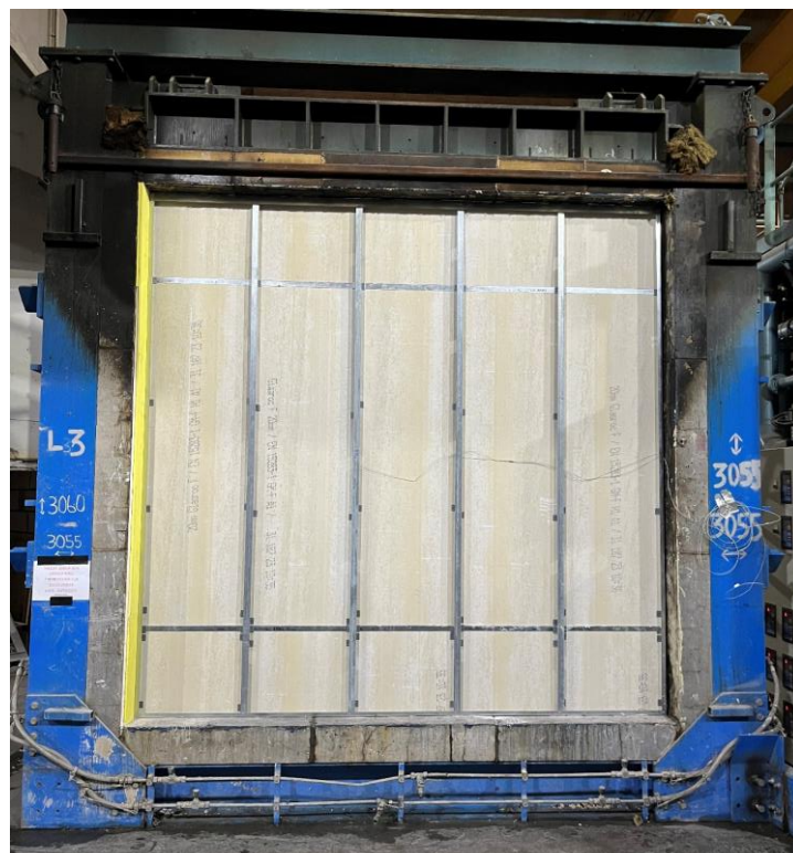
Photo 2 - Specimen during construction - Exposed side boarding view from unexposed side. Note the angles on the horizontal joints.
