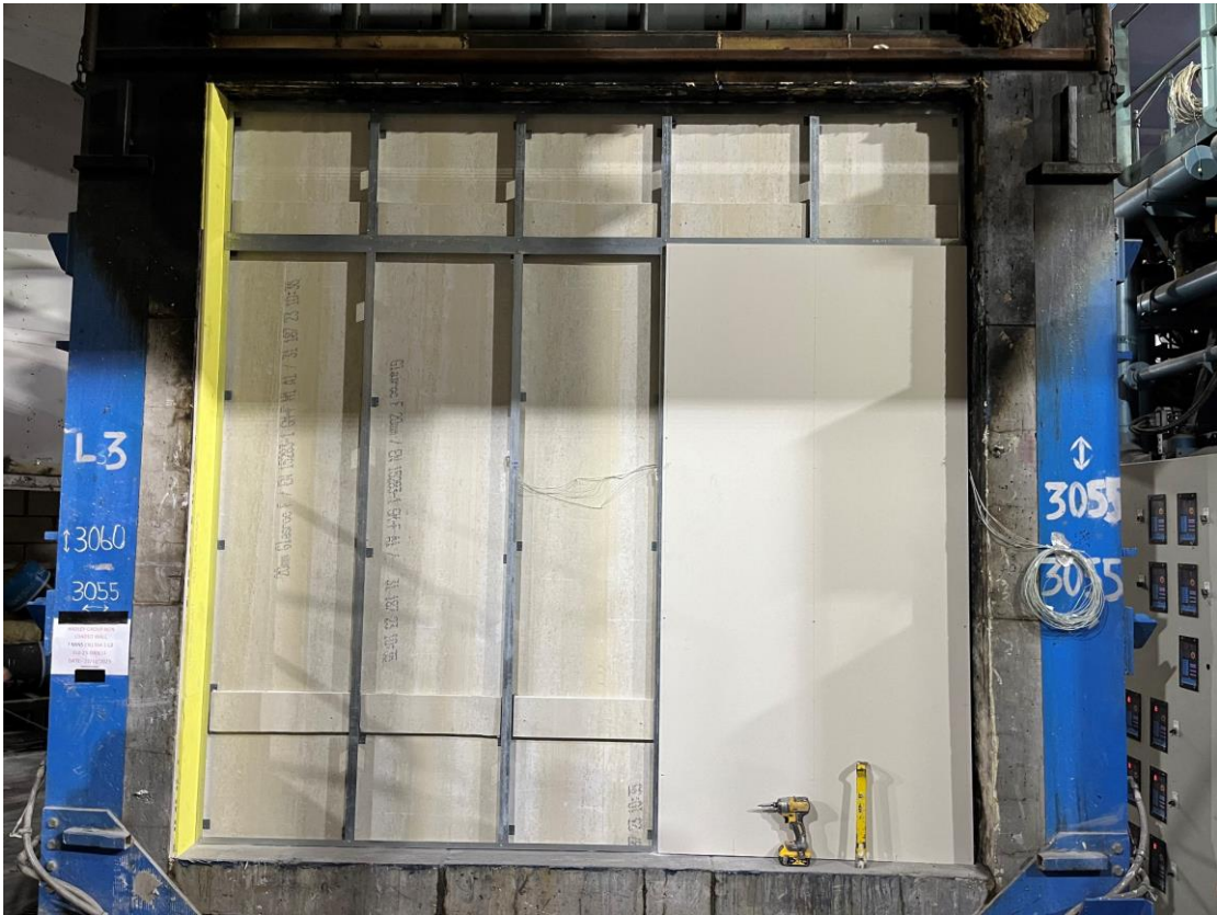
Photo 3 - Specimen during construction - Unexposed side boarding – first layer. Note the boards over the angles on the horizontal joints.
