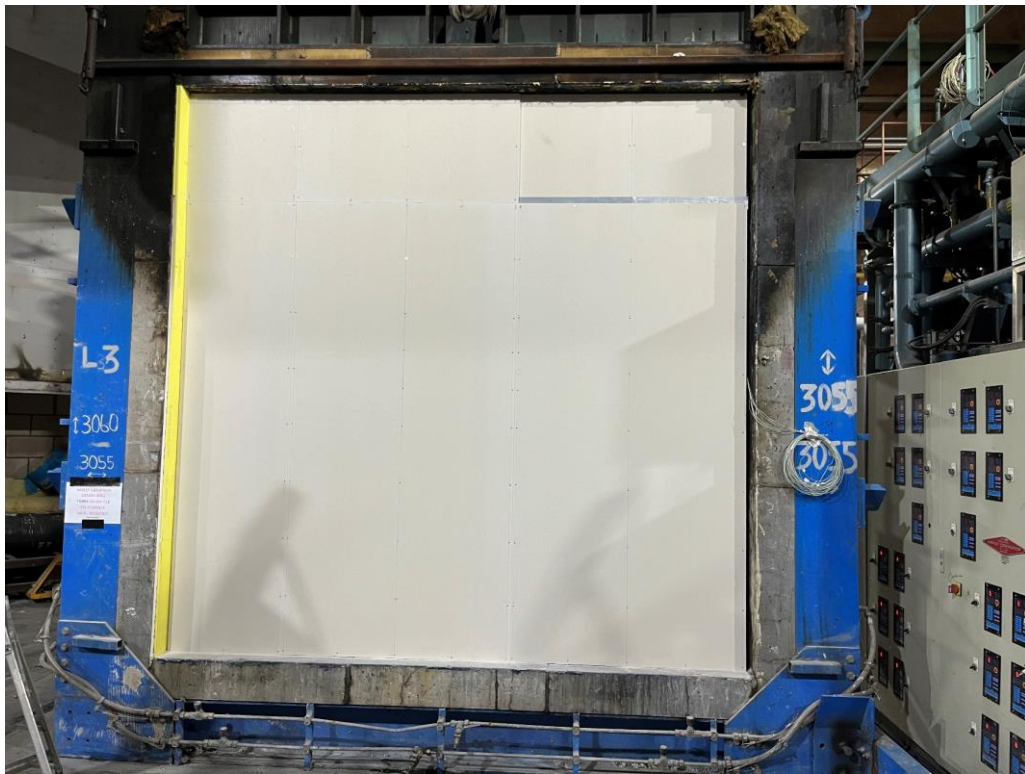
Photo 5 - Third layer of boarding on the unexposed side. Note the fixing strap.
